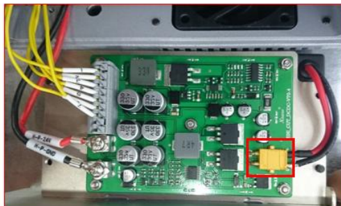
12, Connection the power like picture show then put back the Mainboard and fix it well
